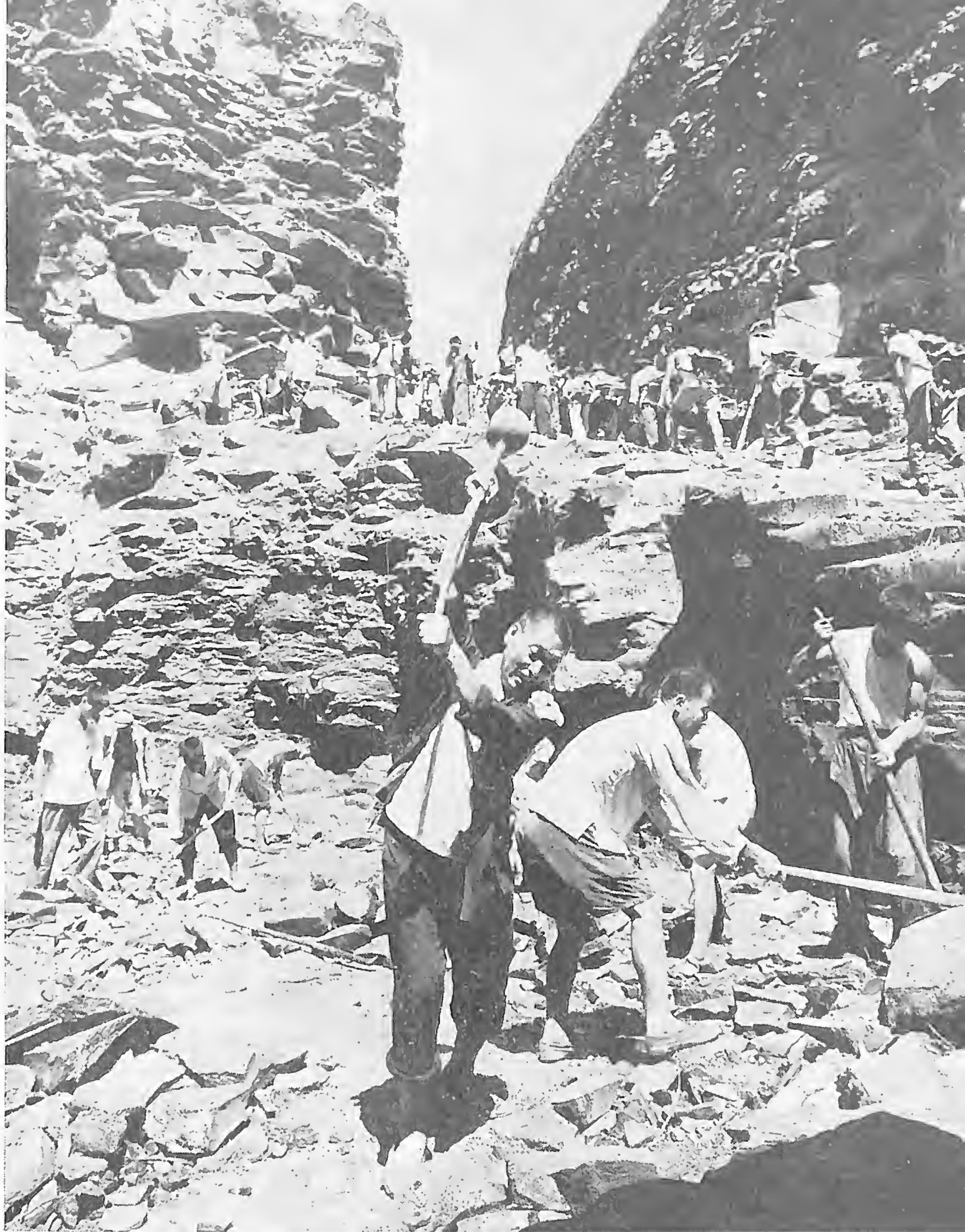
Members of the Niehebia brigade, Penglai county, Shantung province, dig an irrigation well with their own forces.
